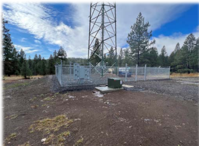
Pictured: AT&T FirstNet tower in Camp Sherman.
